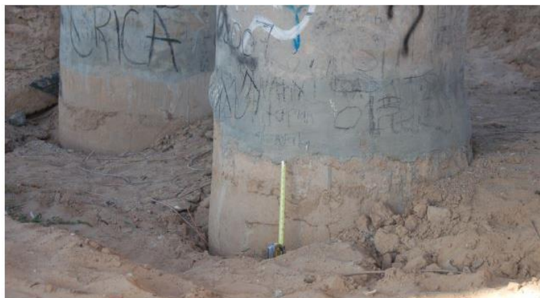
Figure 9.36: Photo at Bent 6 of Felipito Highway Bridge showing 30 to 50 cm of vertical displacements following soil liquefaction (from Turner et al. 2014).
